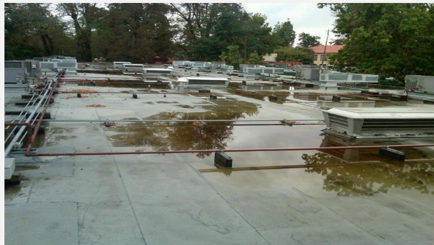
Roof structure failing
