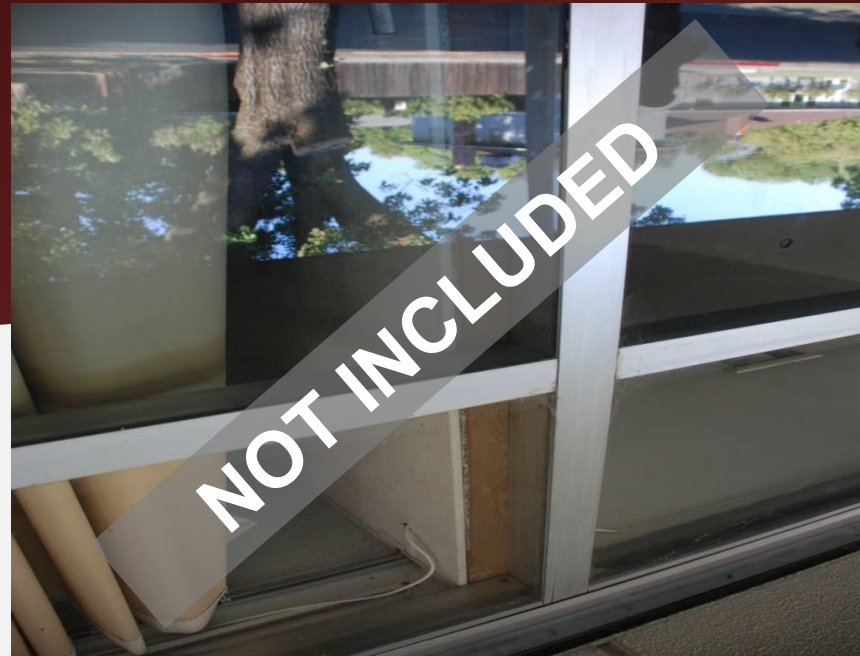
No finish at interior wall
