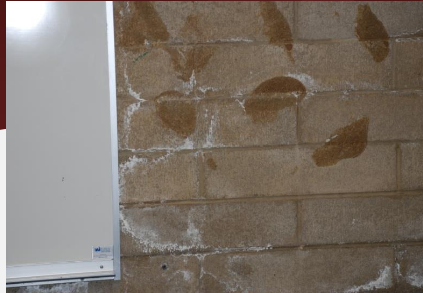
Water intrusion in science classrooms
