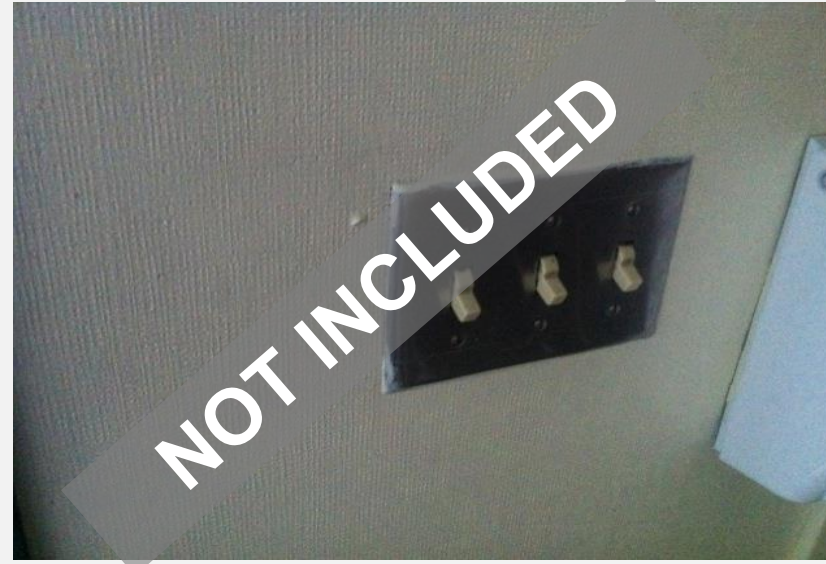
Inefficient energy lighting controls
