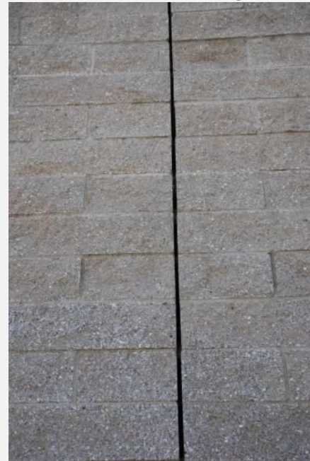
No caulking or sealant at joints
