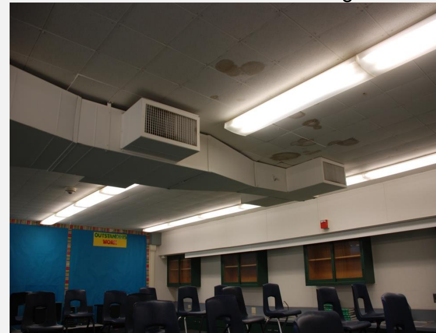
Water intrusion/inefficient air distribution
