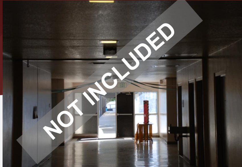
Poorly lit hallways
