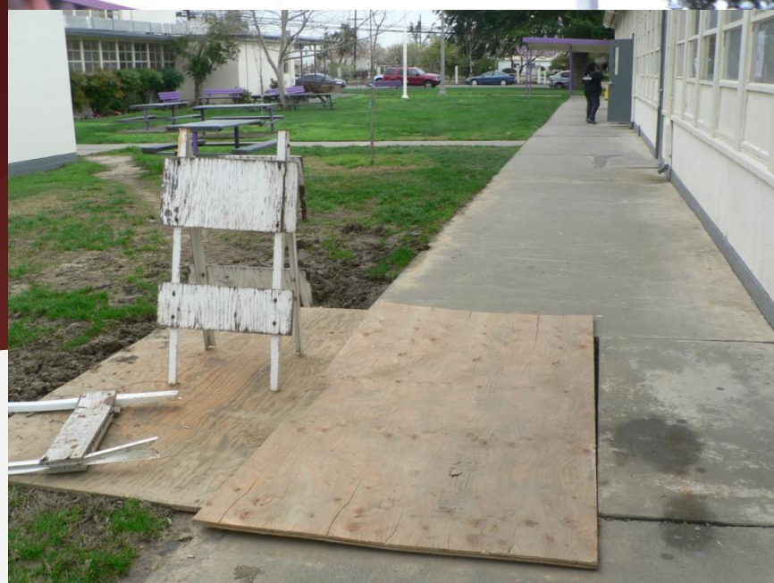
Hole at concrete walk
