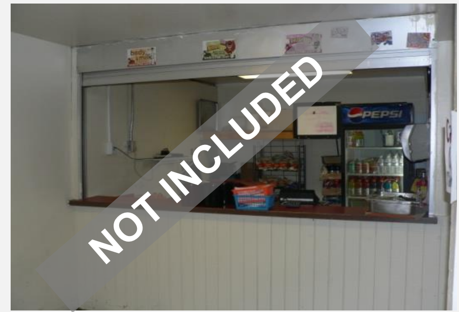
Inadequate kitchen facility
