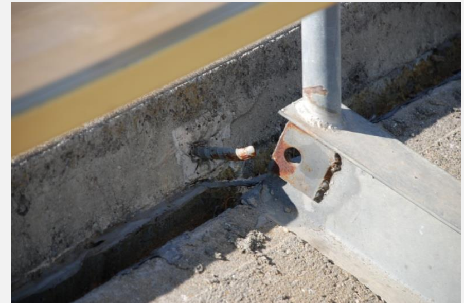
Exposed rebar at stadium
