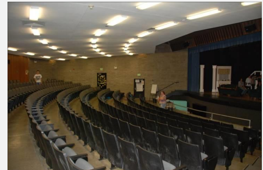
Lack of wing space, theatrical lighting, catwalk and ADA access
