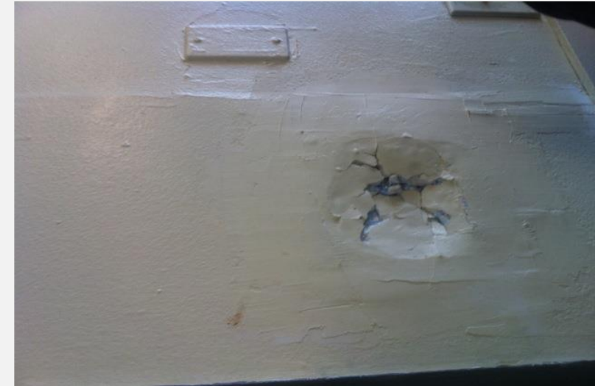
Holes in walls
