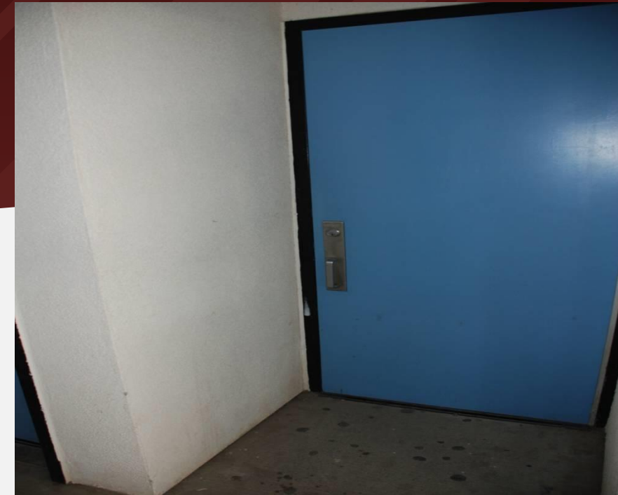
Non-ADA compliant door
