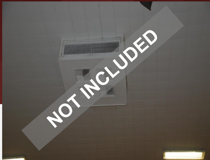
Inefficient distribution of air in gymnasium and water intrusion
