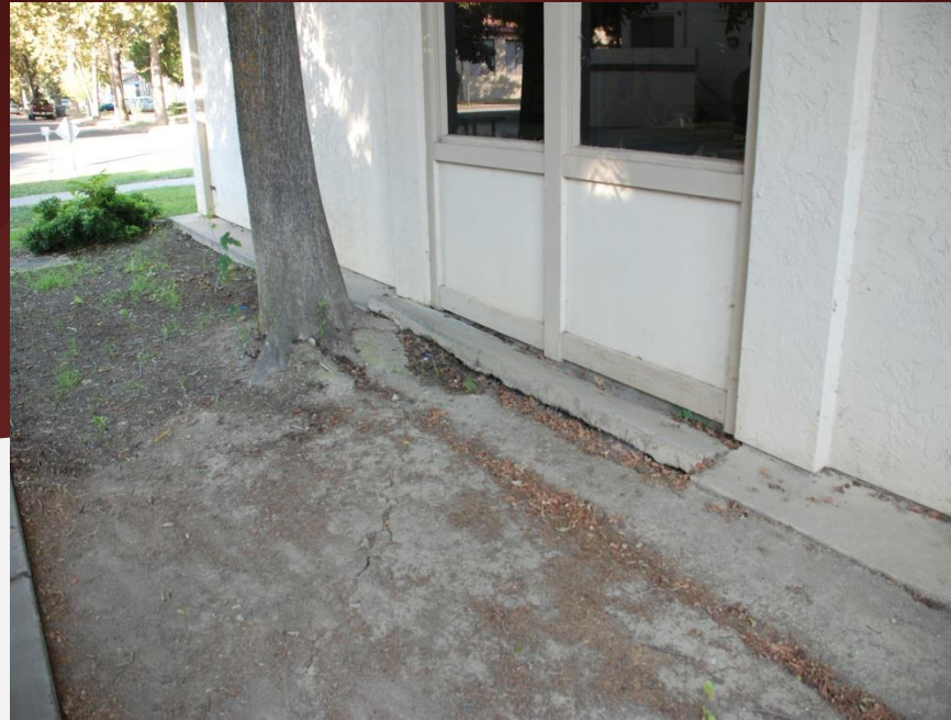
Heaved concrete at building
