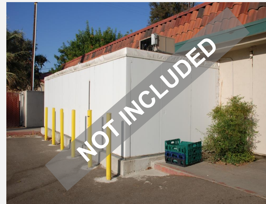
Exterior exposed coolers and freezers do not meet DSA requirements for restraint of walls
