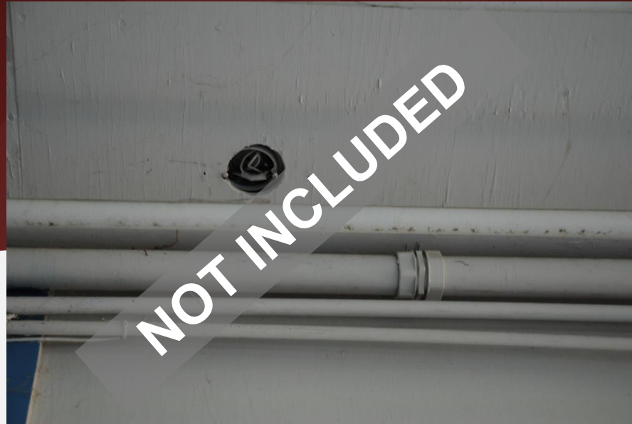
Exposed electrical wires
