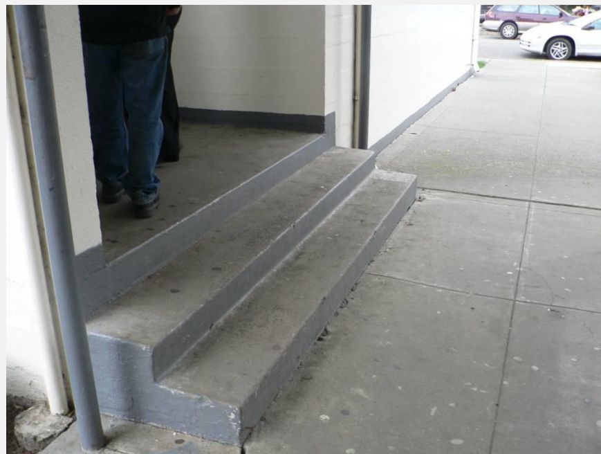
No handrails provided
