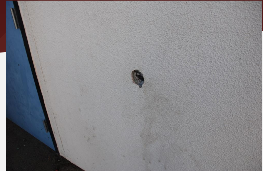
Hole in exterior plaster
