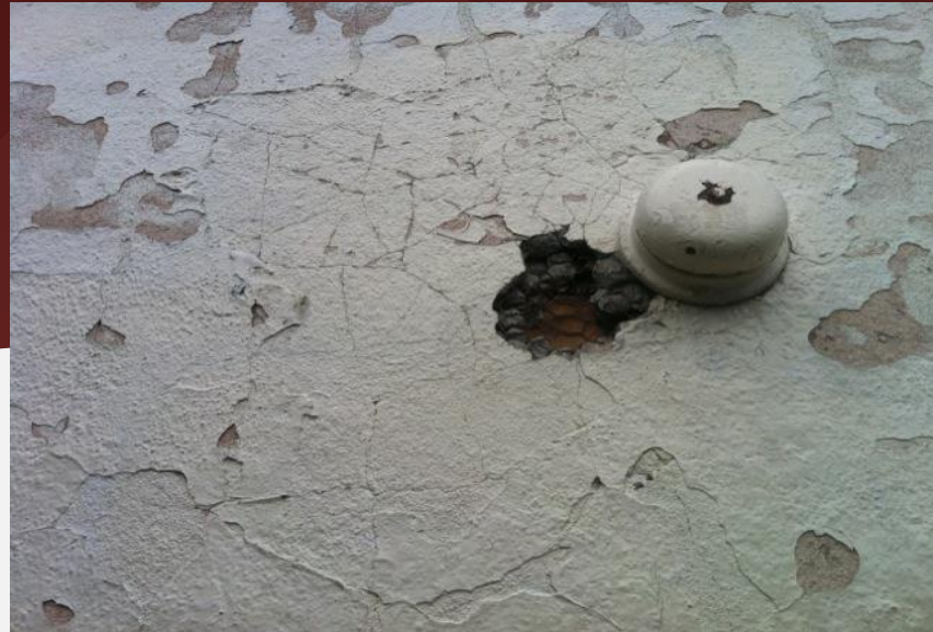
Holes in exterior walls and deteriorated plaster
