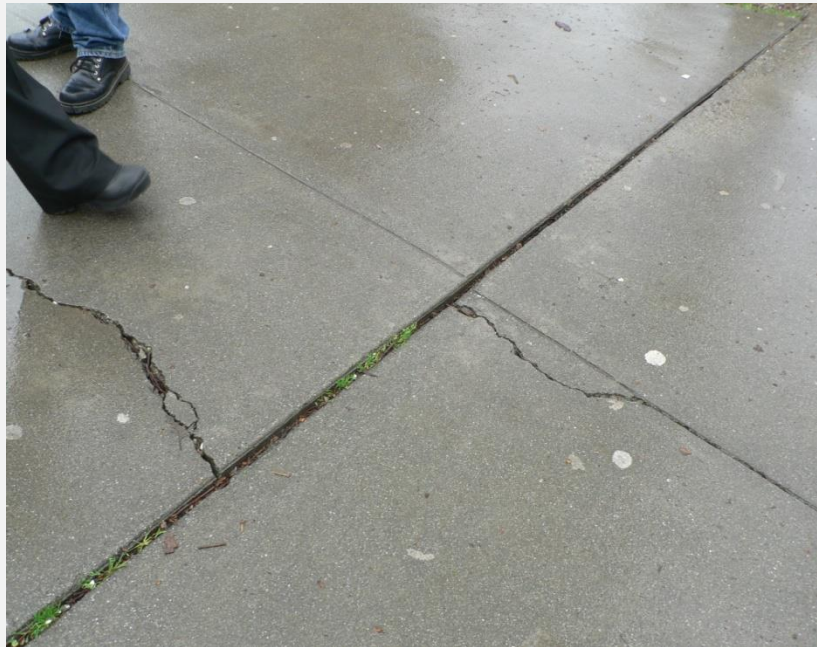
Cracked and unlevel concrete
