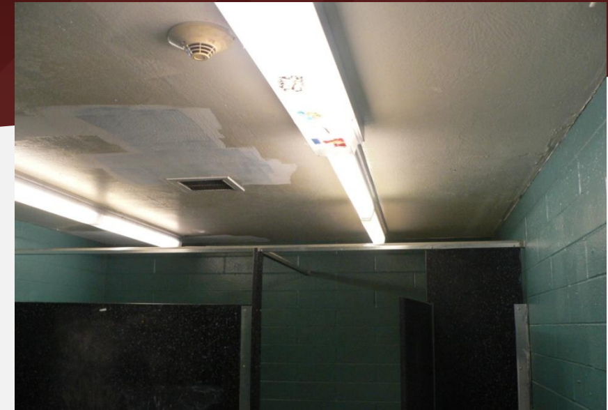
Restroom with water intrusion
