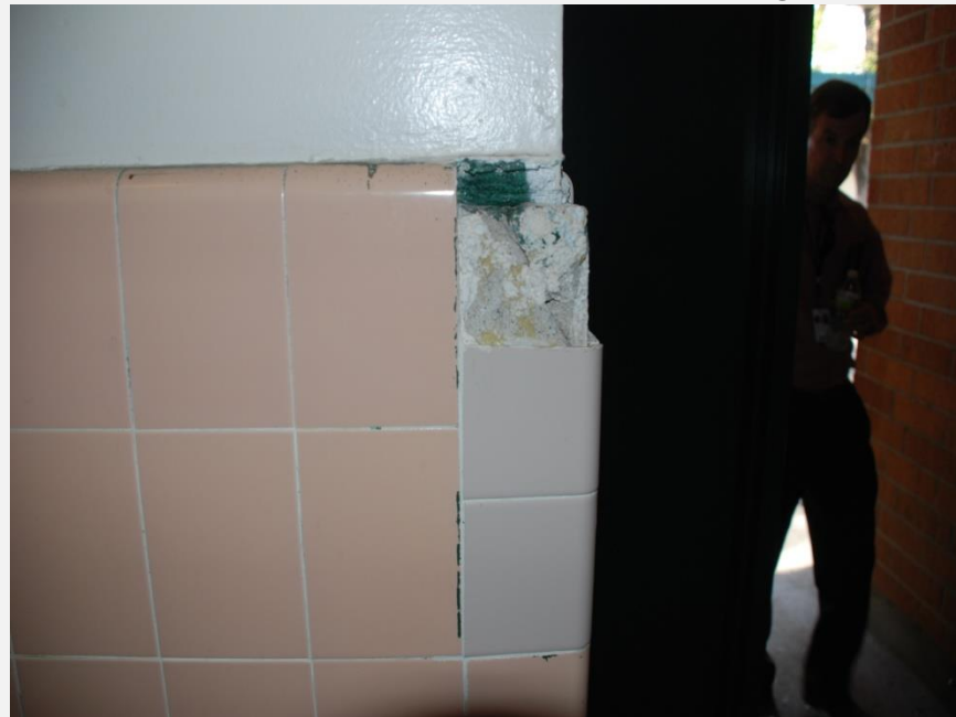
Broken missing tile
