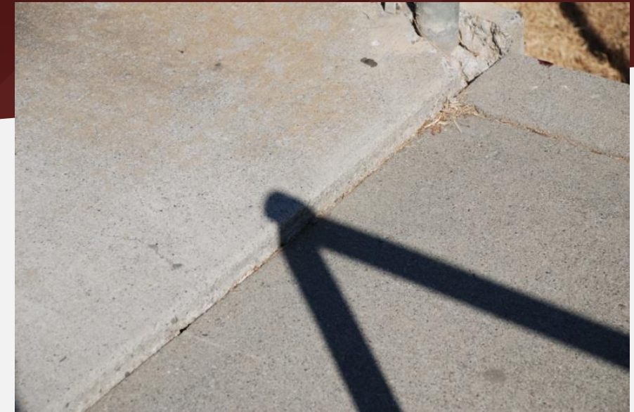
Heaved concrete at stadium
