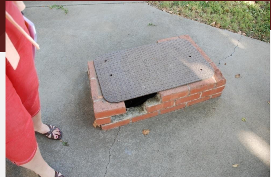
Electrical vault with exposed wires
