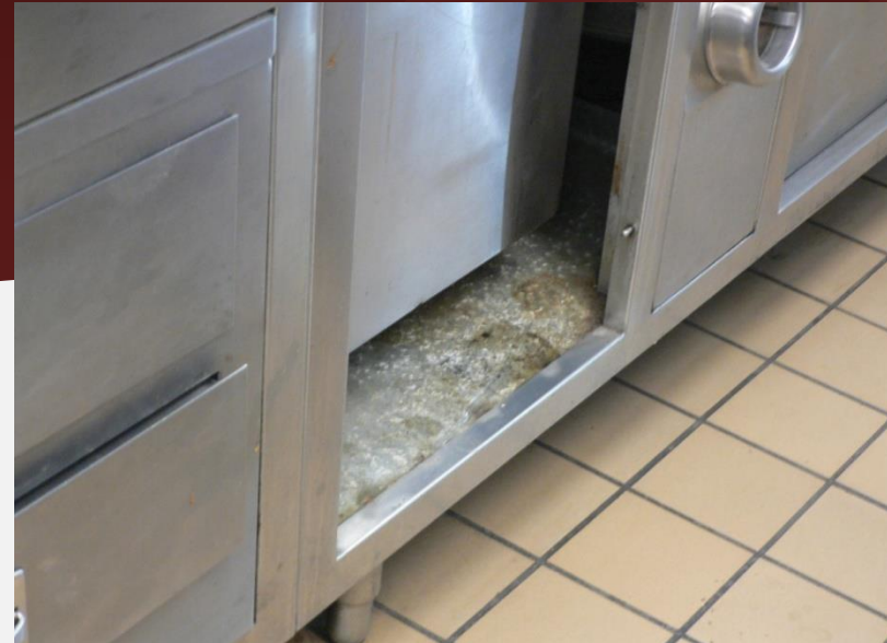
Existing kitchen mold issue
