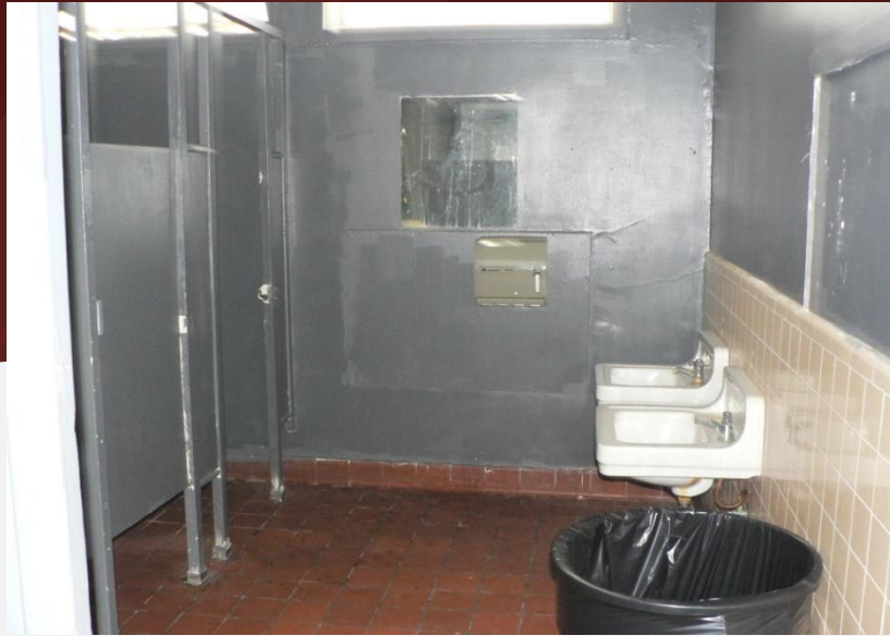
Deteriorated walls at restrooms
