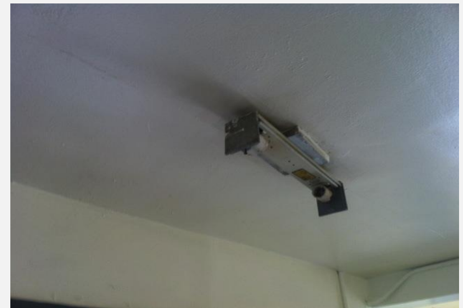
Inefficient / no lighting
