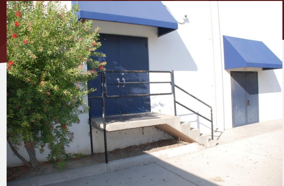
Non-ADA accessible doors/stairs
