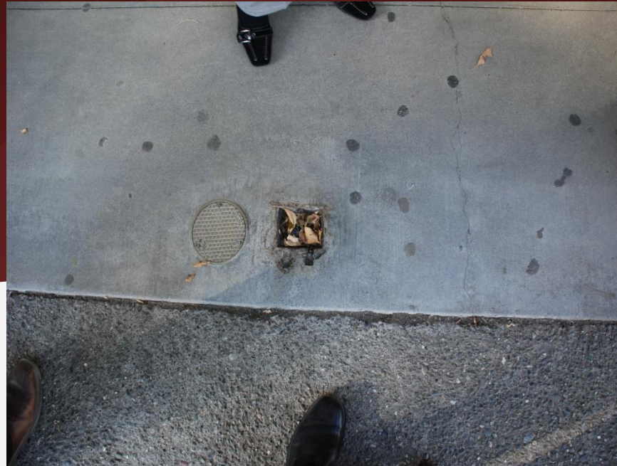
Tripping hazard at sidewalk
