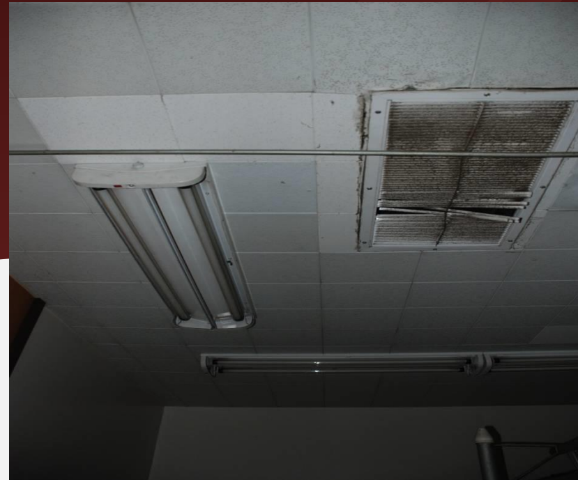
Hazardous/dirty conditions at kitchen
