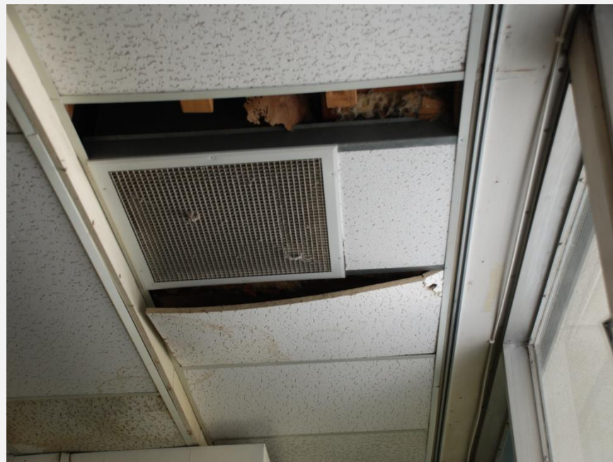
Deteriorated ceiling conditions
