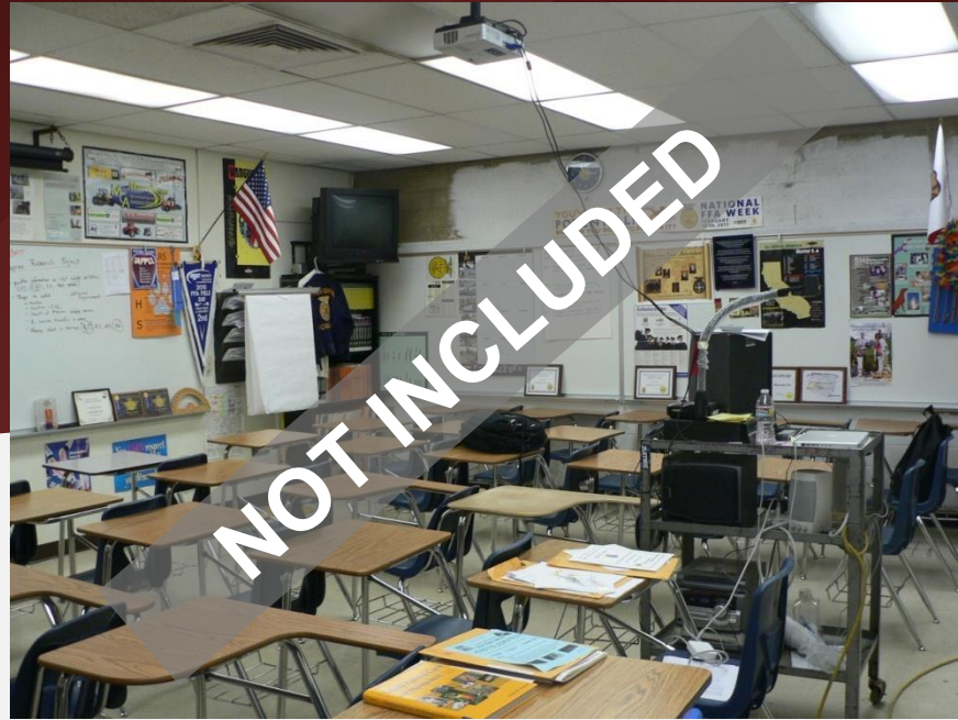
Improper wiring for technology
