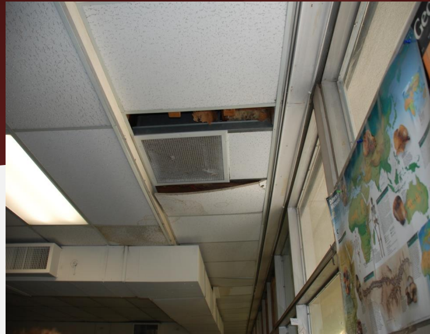
Water intrusion at ceiling
