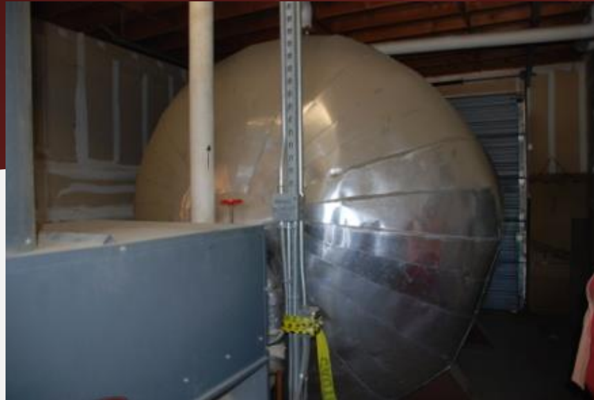
Outdated inefficient boiler
