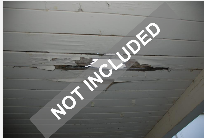
Failing deck at covered walking
