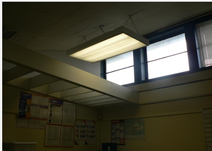
Poor or inadequate lighting
