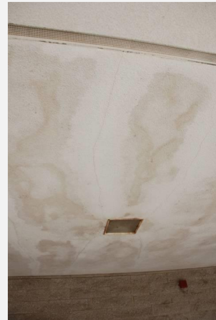
Water intrusion at ceiling
