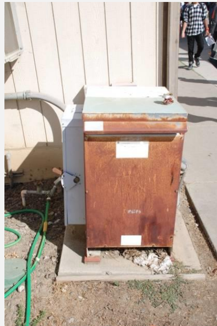
Exposed high voltage transformer
