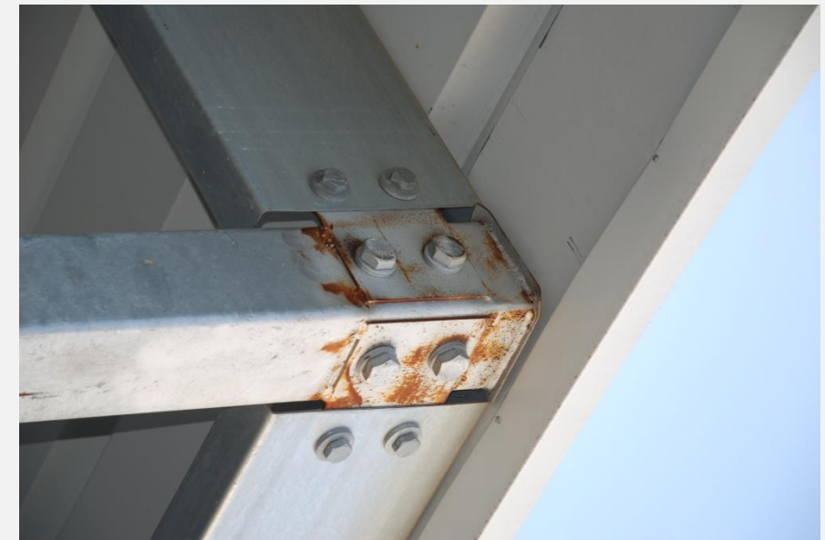
Rust at steel canopy
