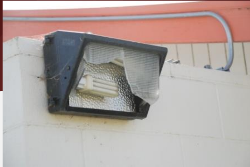
Broken lighting at stadium
