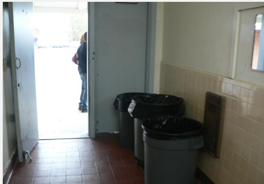
Non-ADA compliant doors
