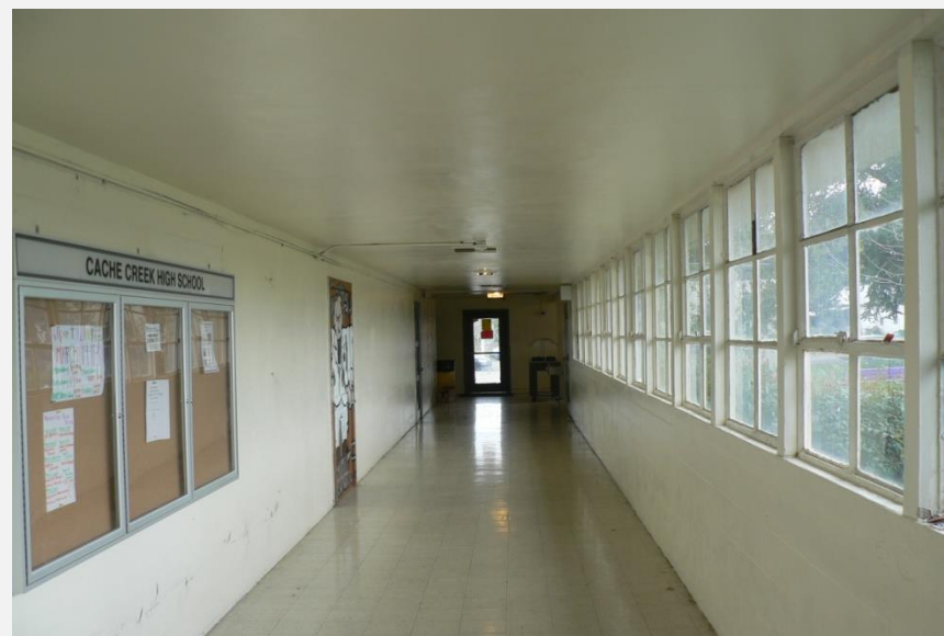
Inefficient windows and leaking roof
