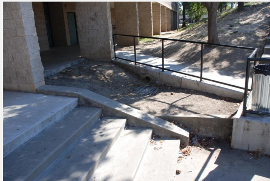
Non-existing. landscaping / lack of handrails
