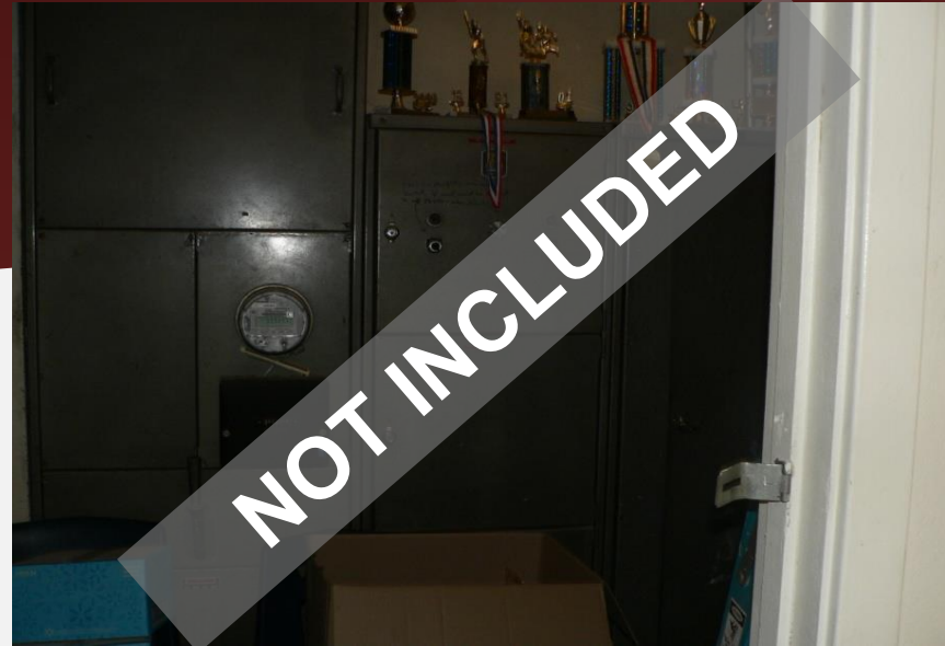
Trophies displayed on electrical equipment
