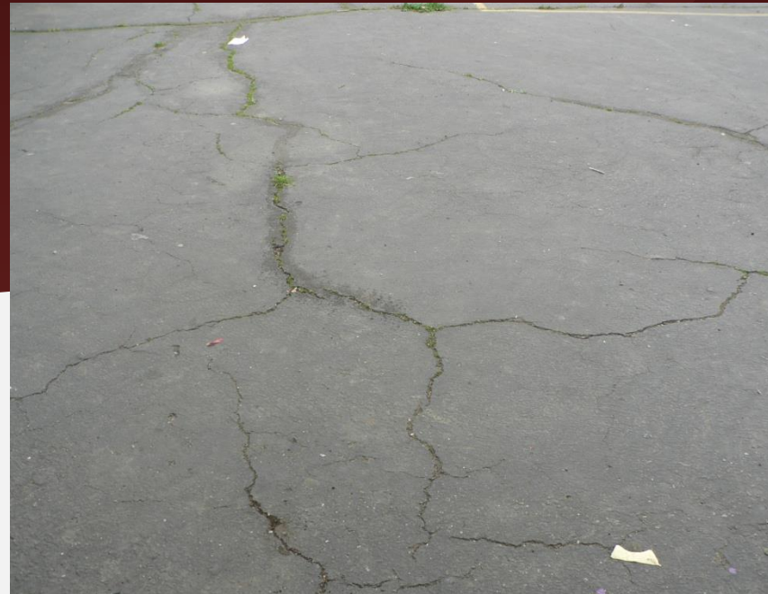
Cracked and deteriorated paving
