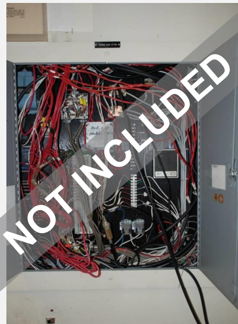
Wire management issues
