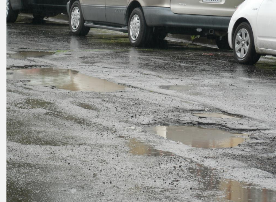
Potholes at paving
