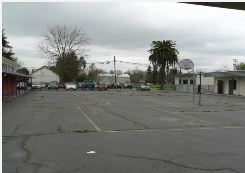
Asphalt needs replacing
