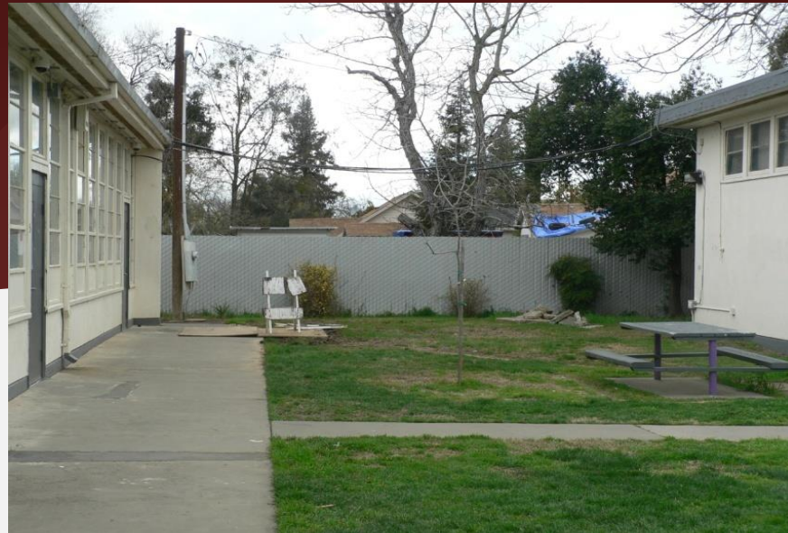
Poor / Non-existent drainage
